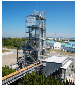
Carbon Capture Pilot Plant
