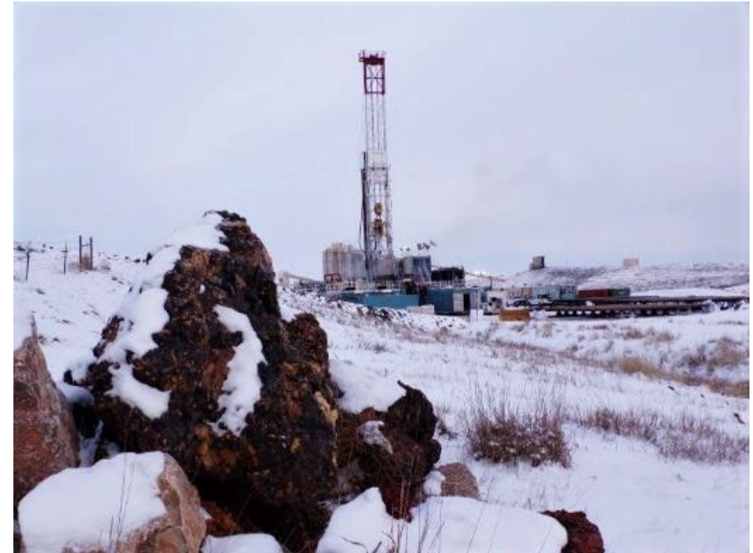
Drilling the University of Wyoming's test CO2 sequestration well under DOE's CarbonSAFE program in 2022.
