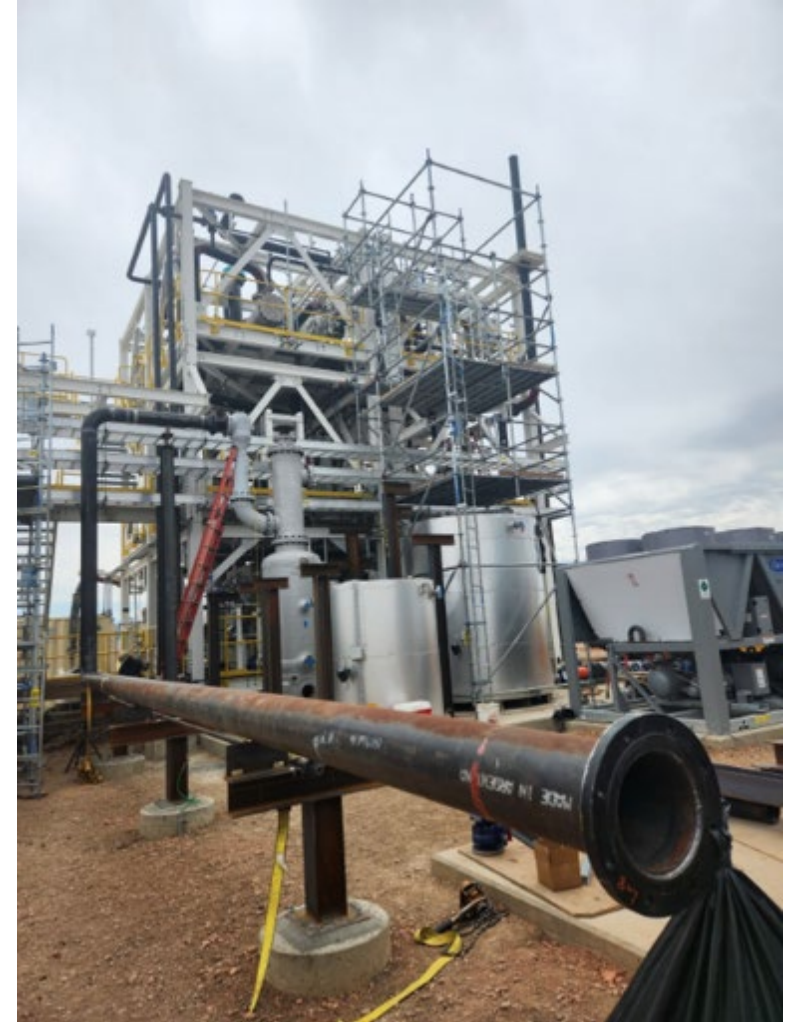
KHI's solid sorbent test facility under construction in August 2023 at the Wyoming ITC
