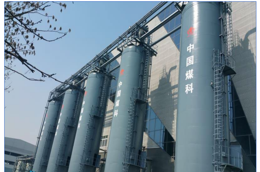
Coal Powder Silo for High-Efficiency Coal Powder Boiler
