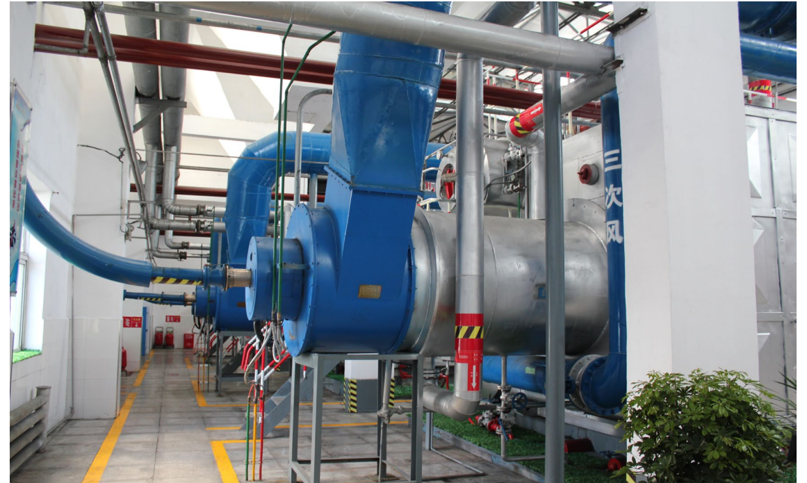
Interior view of efficient coal powder industrial boiler
