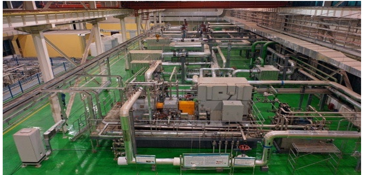
China's first large-scale 5-megawatt supercritical CO 2 cycle power generation experimental unit
