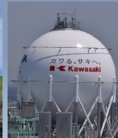
Japan's largest liquefied hydrogen tank (Kobe Liquefied Hydrogen Loading Terminal)
