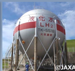
Liquefied Hydrogen Tank (Tanegashima Space Center)
