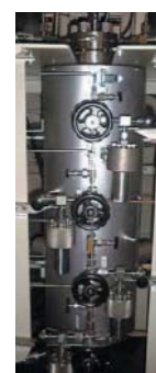
Photo 2 Solid-liquid separation unit
