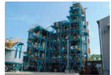
Photo 2 Pressurized, two-stage gasification plant
