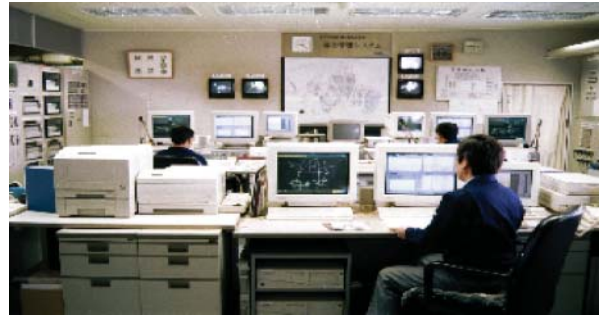
Centralized monitoring and control room
