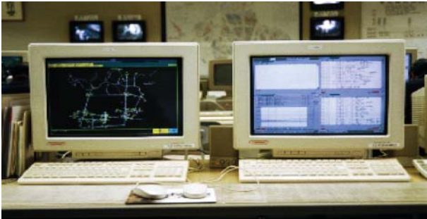
Centralized monitoring computers
