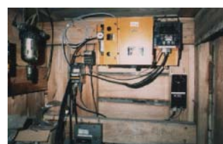
Gas drainage monitoring sensors
