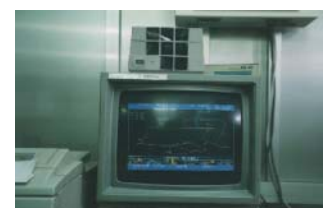
Gas drainage monitoring computer
