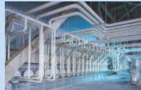
Flue gas desulfurization facility
