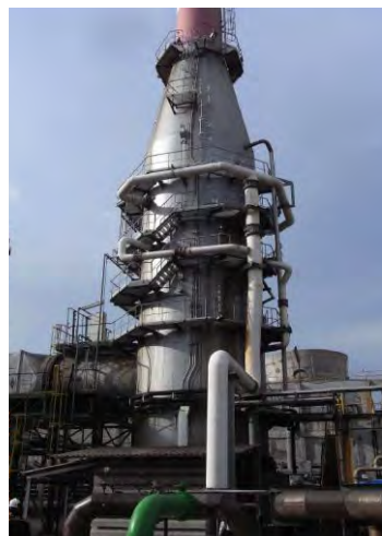
54MW Power Plant in Thailand
