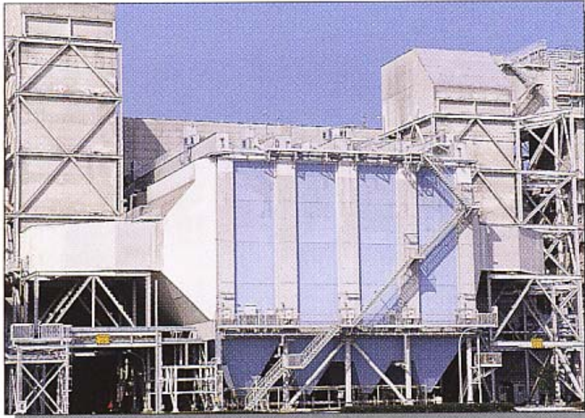
Matsuura Thermal Power Station
